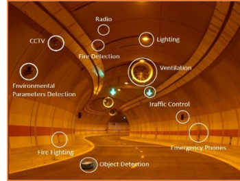
Electro Mechanic & Control System
